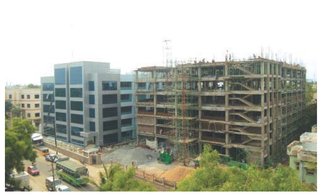
The emerging new building for IP and surgical theatres at Aravind-Madurai, adjacent to the newly inaugurated Dr. G. Venkataswamy Eye Research Institute
